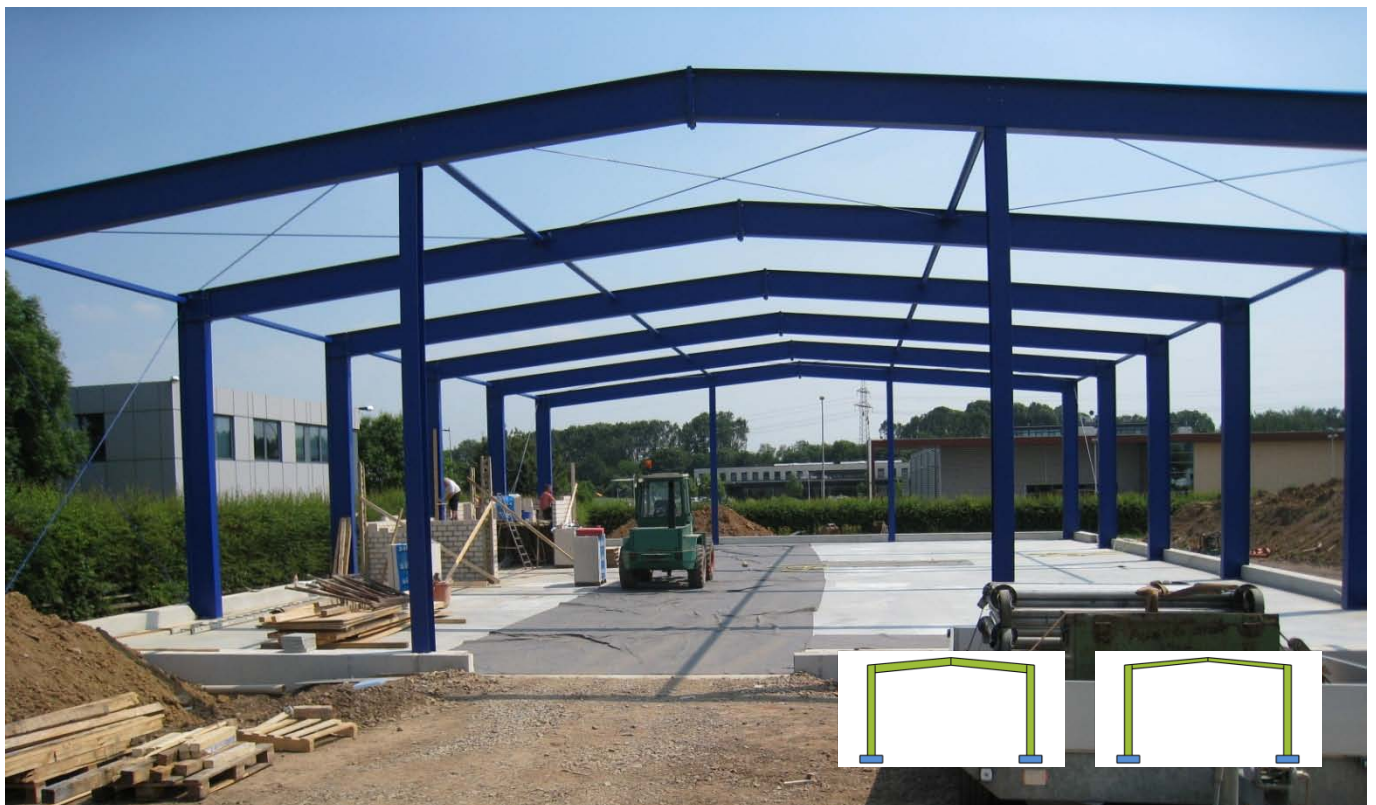
Figure 4: Single storey building with a steel frame, symbols for steel frame in grade S 235 (left) und grade S 460 (right)
